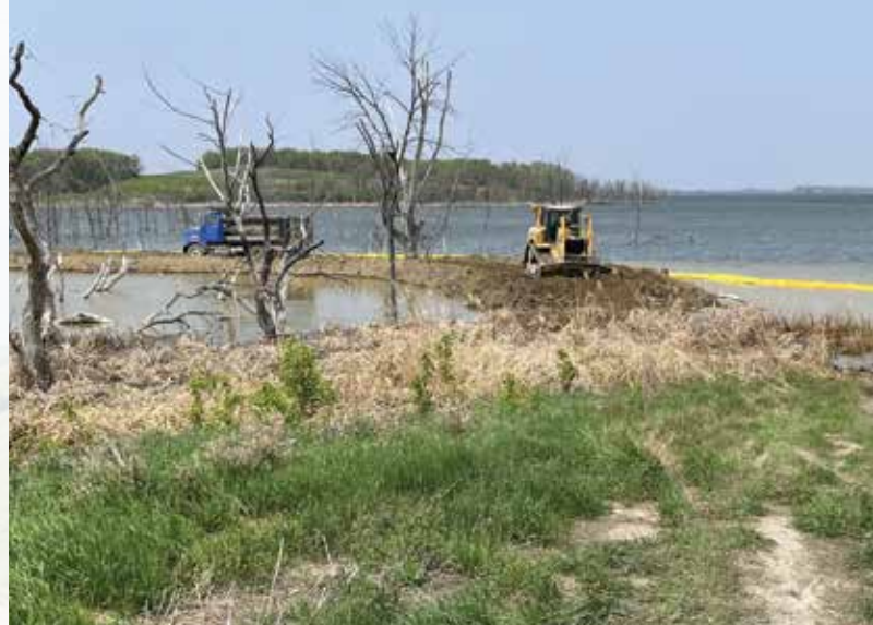
The early stages of construction in building a safe public access to the Engel's Point Wildlife Management Area.
