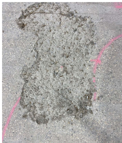
Figure 1: Example of an exposed delaminated area inside a larger spray-painted boundary
