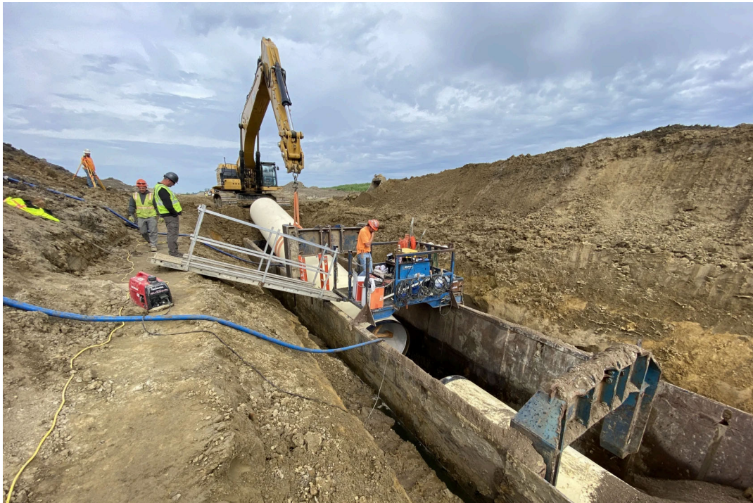
A crew works on installing pipeline for the Red River Valley Water Supply Project. Contributed / Garrison Diversion Conservancy District
